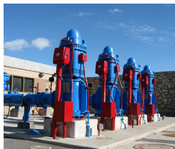
Davis Pump Station
