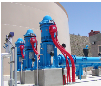
Piedmont Pump Station
